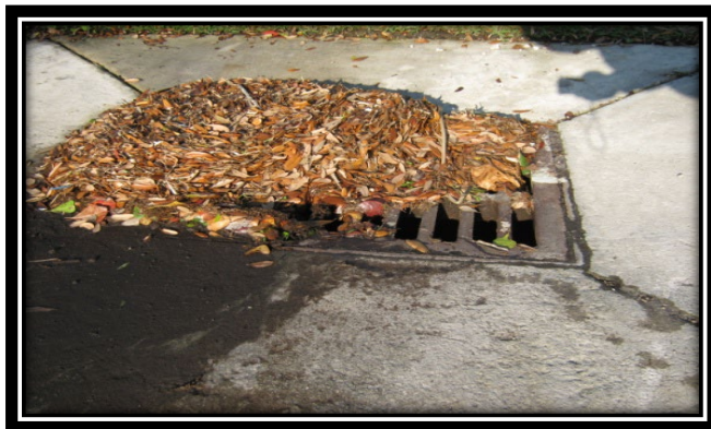
Storm Drain Blockage
