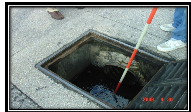
Missing Pollution Retardant Baffles
