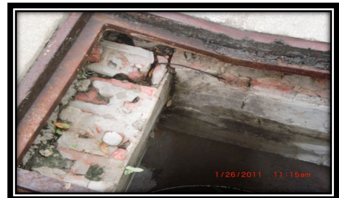
Concrete Repairs Required Inside Catch Basin
