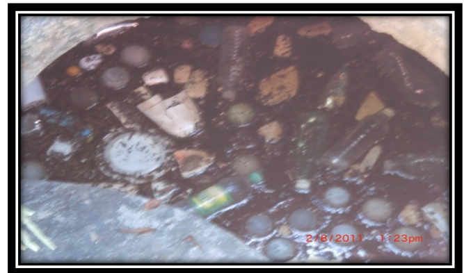
Debris & Sediment in Catch Basin
